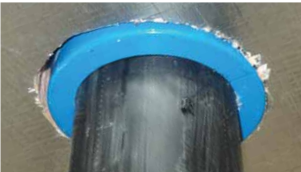
Figure 7 Penetration example - Kingspan Kooltherm® K10 FM G2W White Soffit Board installed tight around the fire collar and HDPE service pipe.
