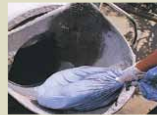
2 Preformulated bags of pigment are added to the concrete truck (one bag per m 3 of concrete).
