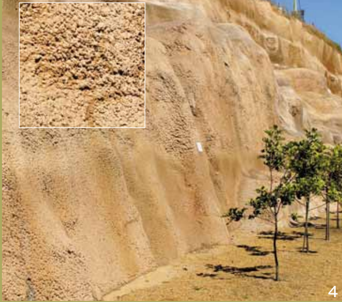
4 Coloured shotcrete is an extremely versatile material for providing wall stabilisation. Varying textures were created by altering the flow of material from the shotcrete nozzle. CCS Suntan was used to colour the concrete.
