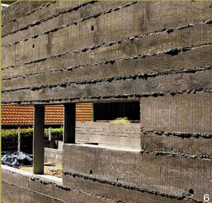
6 A rustic, natural finish complete with authentic timber texture was created using concrete. Oregon timber was used as the formwork. CCS Panther pigment was used to colour the concrete. Architect: Brian Steenbyk.
